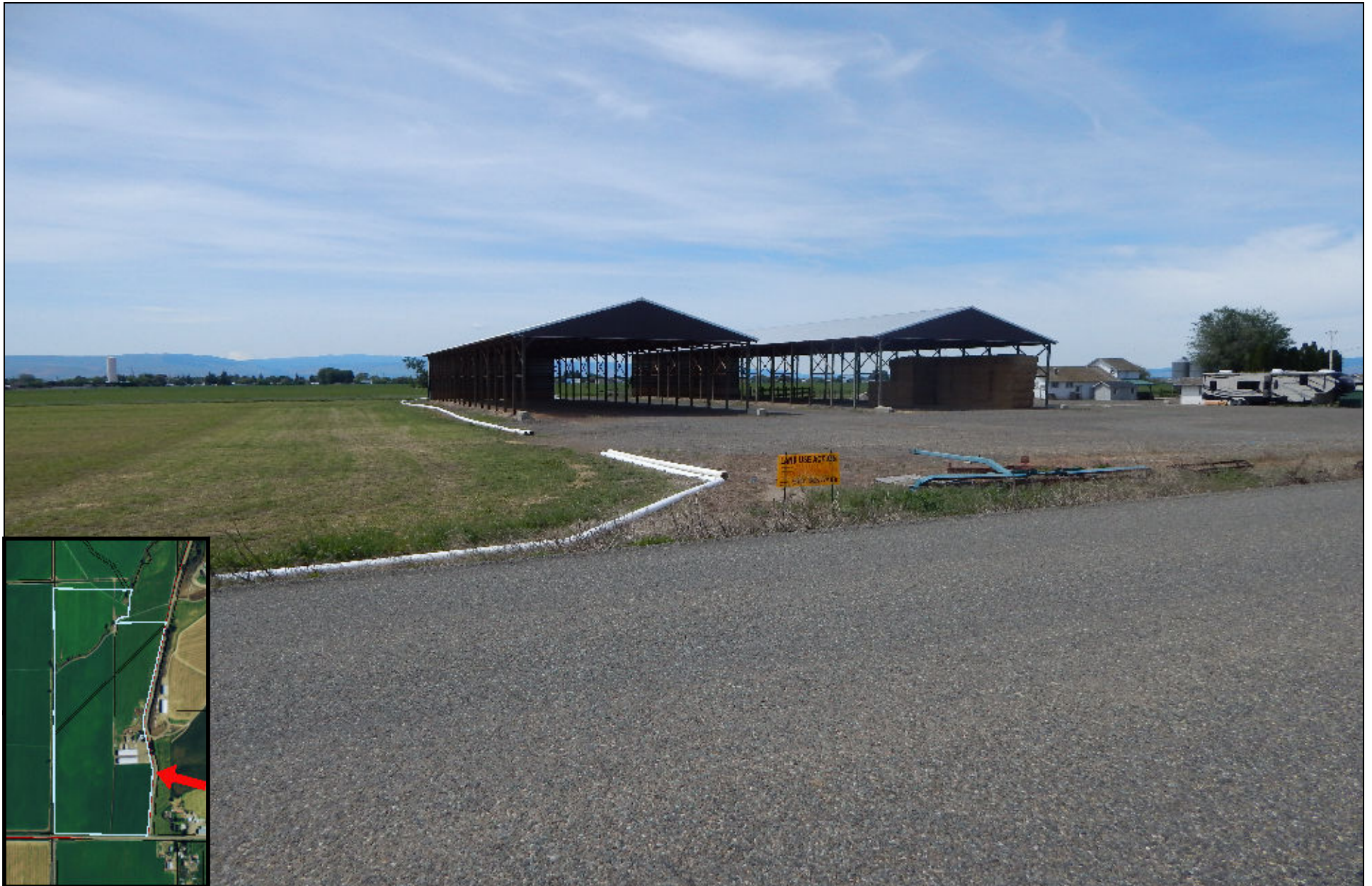
CU-15-00006 Iron Horse Solar Farm
